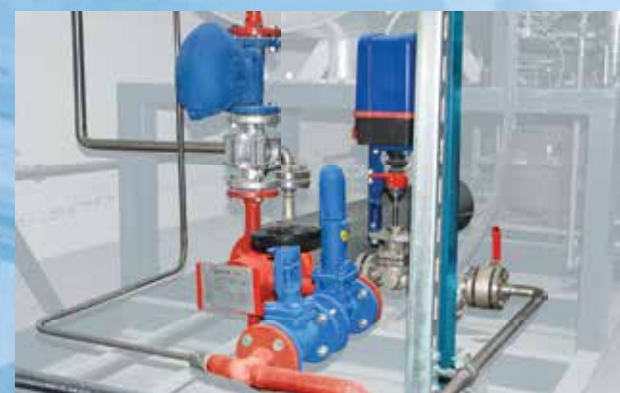
Pressure maintained in a condensate cooler (heat exchanger) belonging to a steam regenerator – improved energy efficiency. Valves: PRESO® or PREDEX® / CONA® / FABAs-Plus / STEVI®
