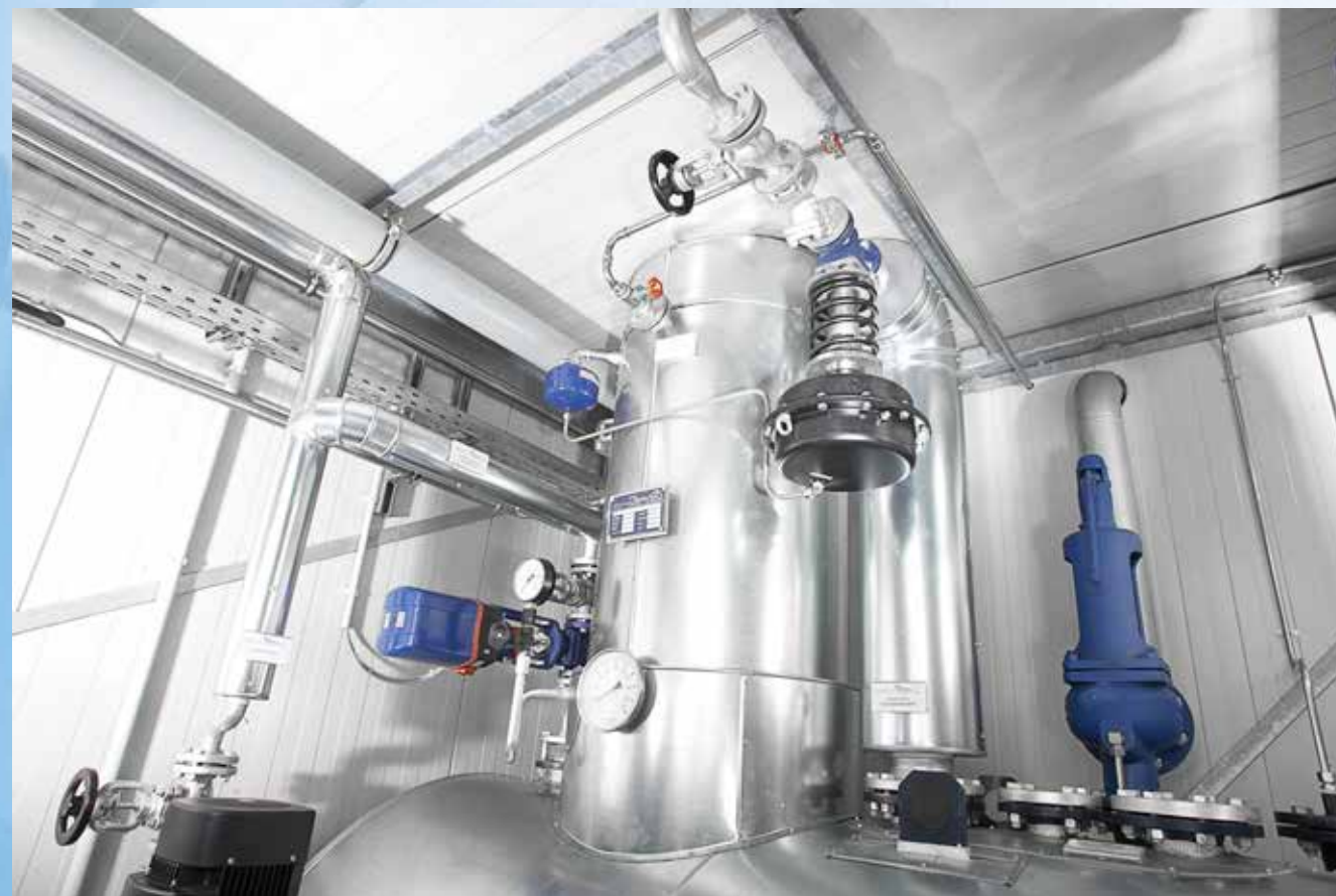
Feed water tank with de-aerator dome. For supplying returned condensate and fresh water to the boiler via the de-aerator dome and the feed water tank
